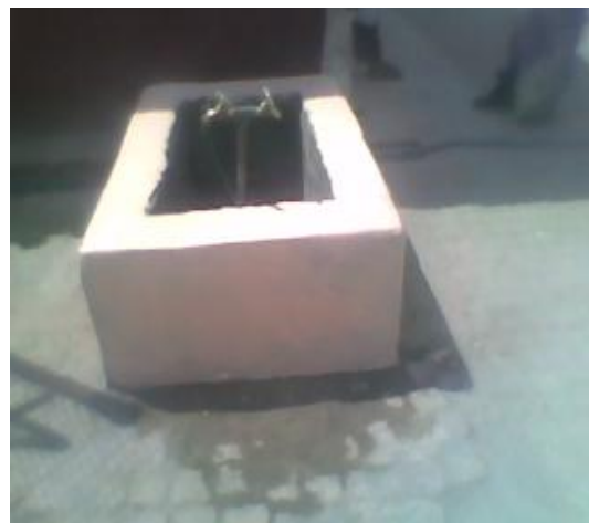
Thutong Primary school securing fixed water pipes after
