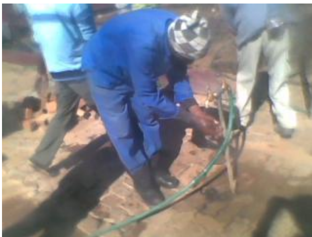
Thutong Primary school water pipe leaking before
